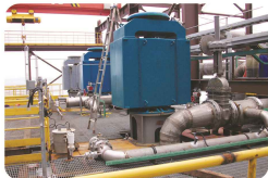
JHB pumps are operating in flue-process at a sulfuric acid plant in Philippines. Capacity: 2400 m 3 /h Head: 25 m
