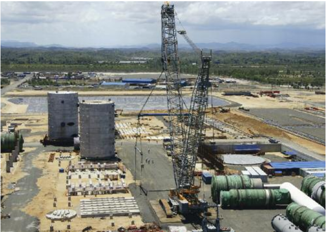
Below: Converter No. 1 in place on site with No. 2 on its way. The mobile 800 t crane can be seen in the foreground.
