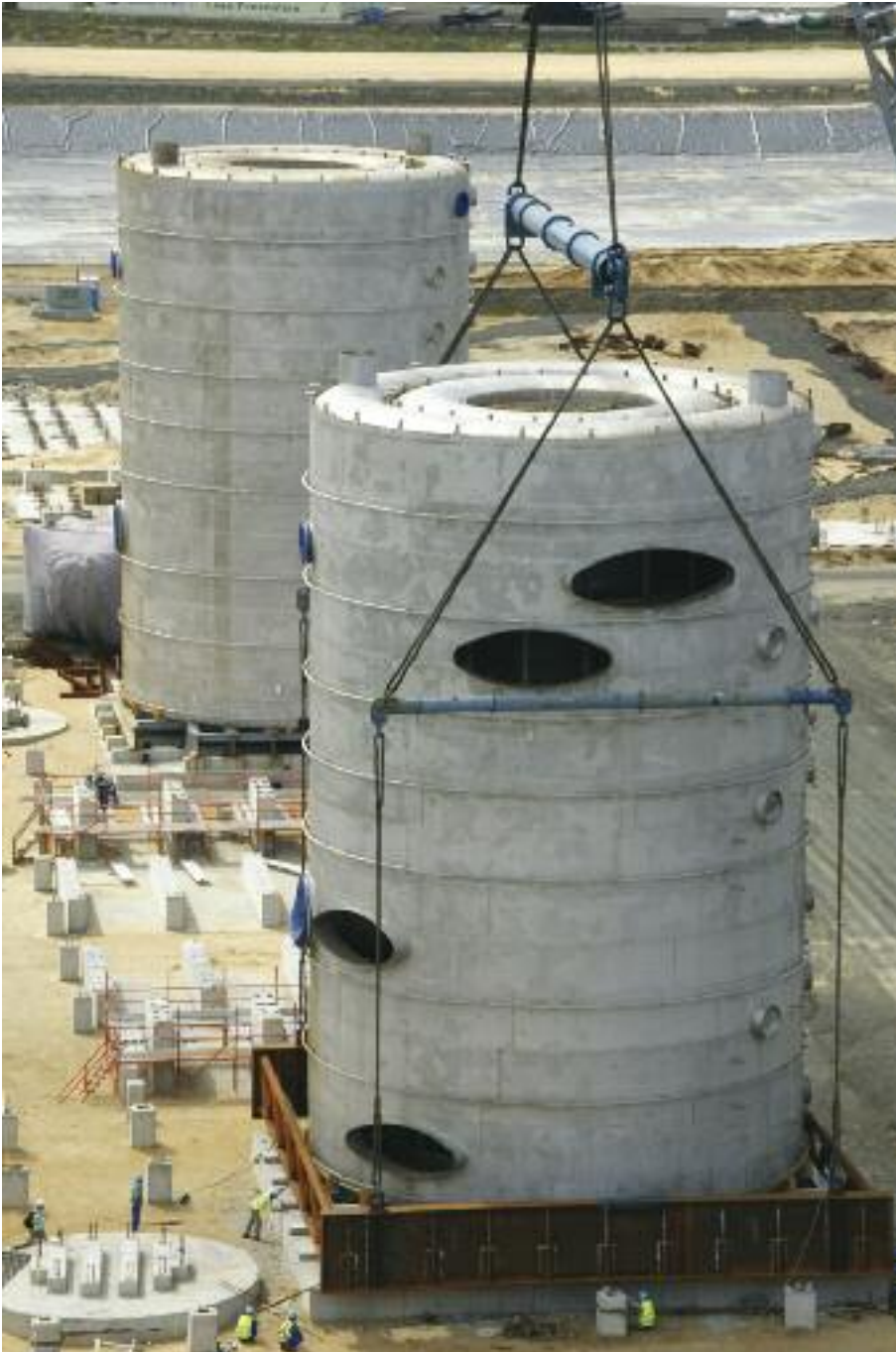
A mobile 800 t crane at site lifted the converters from the SPMT into position onto the foundations.
